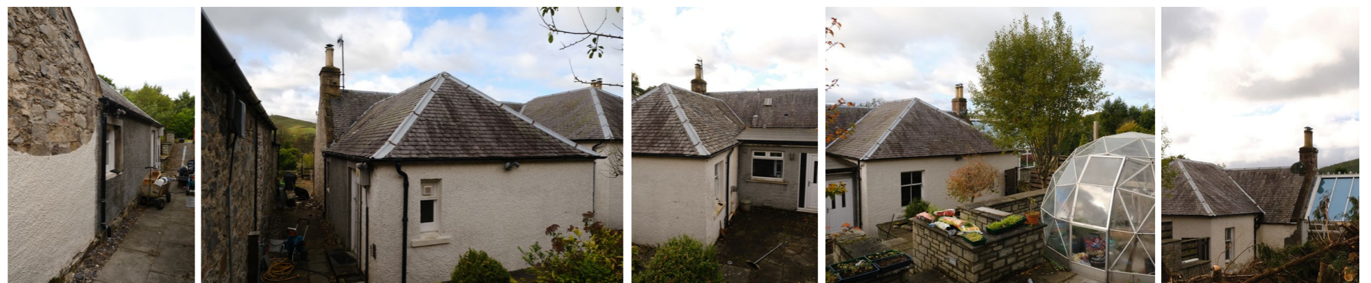
figs. 15-19 Existing cottage - view between Byre and Cottage, kitchen wing and flat roof addition, North elevation with wing to be retained and conservatory.
